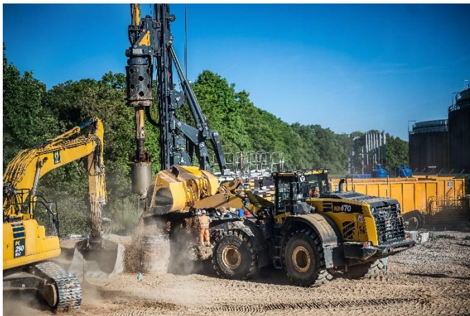
(1) Bauer Resources rehabilitated an area near Duisburg: Using replacement boring, the contaminated soil was replaced with unpolluted material.
